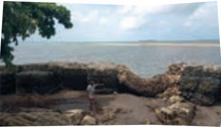
Photo: Breach in the seawall at Walande village, which was constructed in 2022. In the background, you see the remains of the artificial island of Walande, which was the home of Walande people before moving to the nearby mainland of South Malaita in response to several storm events in the early 2000s.
